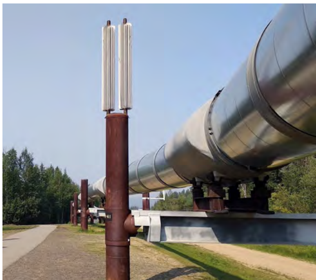
Thermosyphons alongside the Trans-Alaskan pipeline draw heat out of the ground and help keep permafrost temperatures low enough to support the above-ground structure. Alaska pipeline (2019). Photo: Nadezhda Zamyatina/reprinted from ECONOR 2020.
